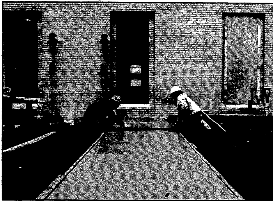
Joe Aquino (left) and Sam Bird, employees of general contractor J.C. Pilato, lay cement Jan. 15 outside the new entrance to what will become a conference facility at the diocesan Pastoral Center in Gates.
