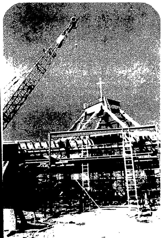
Still a maze of framework and scaffolding, the cross was placed atop the new church April 18, 1979. Turned so that it will be visible from Route 17, the cross was made by parishioners Richard Rodabaugh and Richard Smith.
