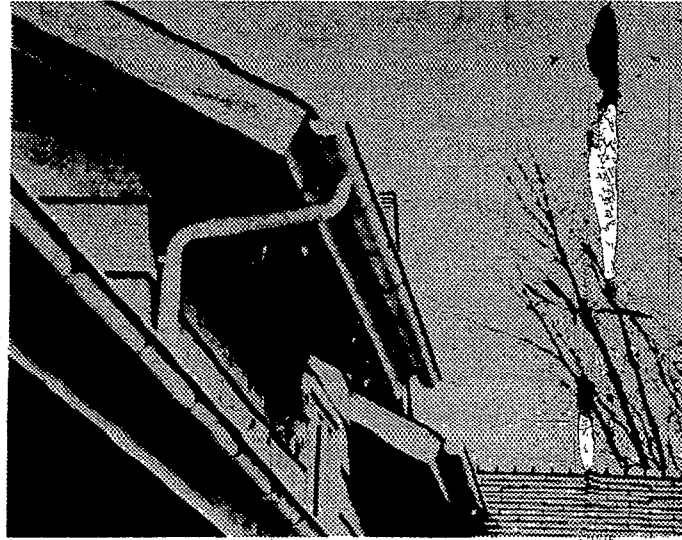
PEELING PAINT under eaves can be corrected by sanding and washing before repainting, say Sherwin-Williams painting experts. Recommended solutions for house paint failures are in a free booklet available at more than 1,500 Sherwin-Williams Decorating Centers nationwide.
